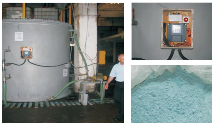
Figure 3. Industrial plant (12,000-14,000 litre tank) for treatment of wastewaters from leather tanning
